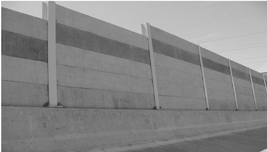
Illustration 18-2: Post-and-Panel Noise Barrier Mounted on Type 7 Barrier: US-6 in Lakewood
